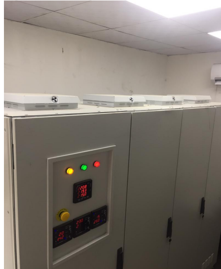
AVR Installed at NCDC-NRL
