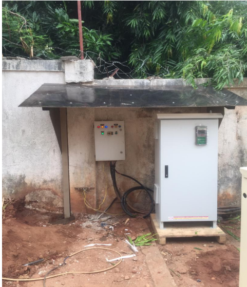
AVR at eHA Residence
